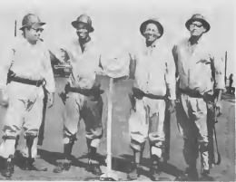
INCREDIBLE ILLUMINATION of some of Lago's far reaches is the project of these four men. They are charged with the installation of low mercury vapor lights...
